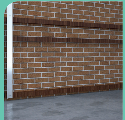
3) Install starter bar, ensuring that it is at least 30mm from the ground.
